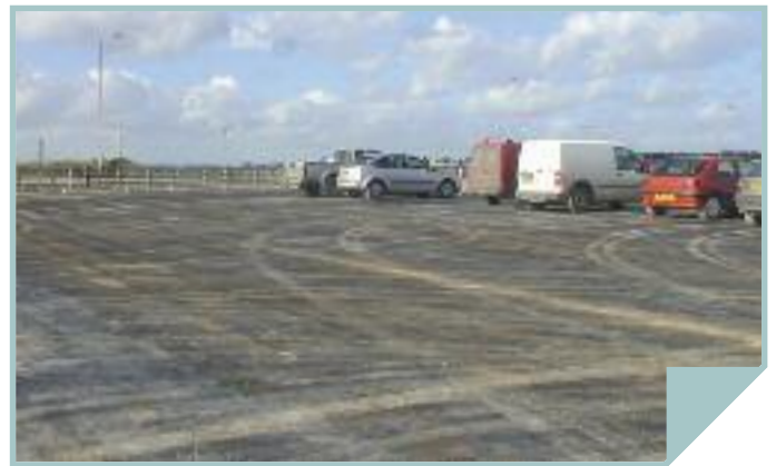
Top: Piling platform after Firmabase treated. Below: Building platform after Firmaroc treated.
